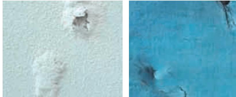
Figure 1: Damage to facades caused by inadequate water vapor permeability
